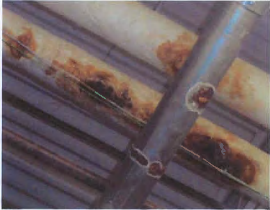
Figure 8 – Chilled Water Piping Leaks and/or Condensation
