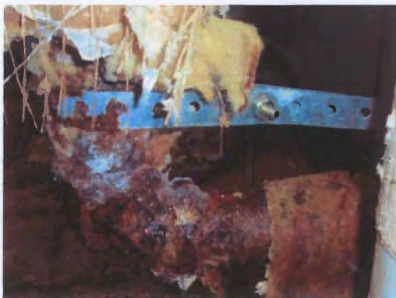
Figure 5 – Chilled Water Piping Deterioration at AHU Connection
