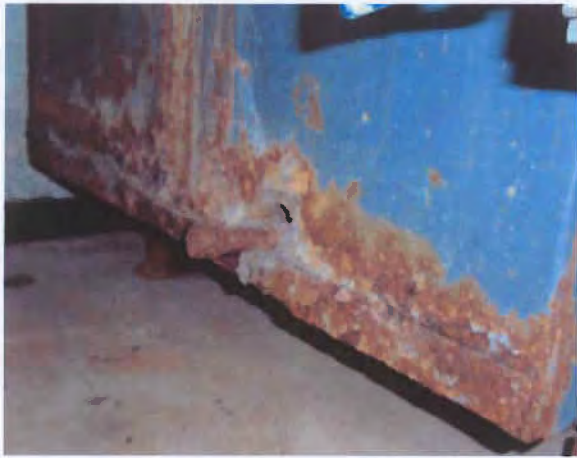
Figure 1 – AHU Casing Deterioration
