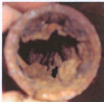
Figure 6 – Chilled Water Pipe Corrosion (Removed by Maintenance Personnel Due to Leak)
