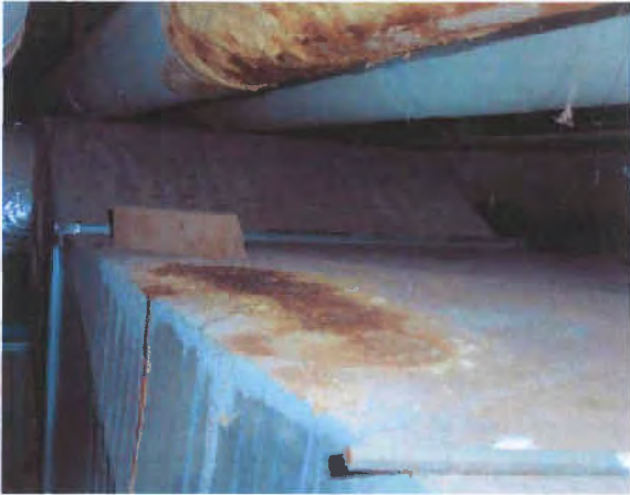
Figure 10 – Chilled Water Piping Leaks/Condensation, Causing Secondary Ductwork Corrosion (Similar Sites Widespread Throughout Building)
