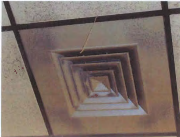
Figure 3 – Smudging of Ceiling at Air Devices, Resulting From Filter Bypass
